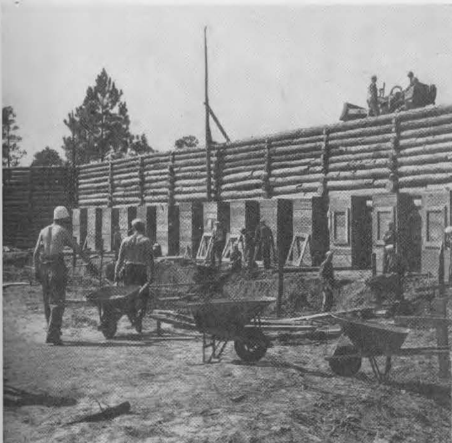
1000 INCH RIFLE RANGE. This was one of the toughest construction projects undertaken by the 83rd at Gulfport. Assertedly a "fool proof" range, this structure called for sand-bagged firing pits, an 18-foot parapet of logs backed by a compacted earth fill. When completed, after several weeks of hard work, our Seabees posted a sign which read—"Constructed by the 83rd Battalion."
