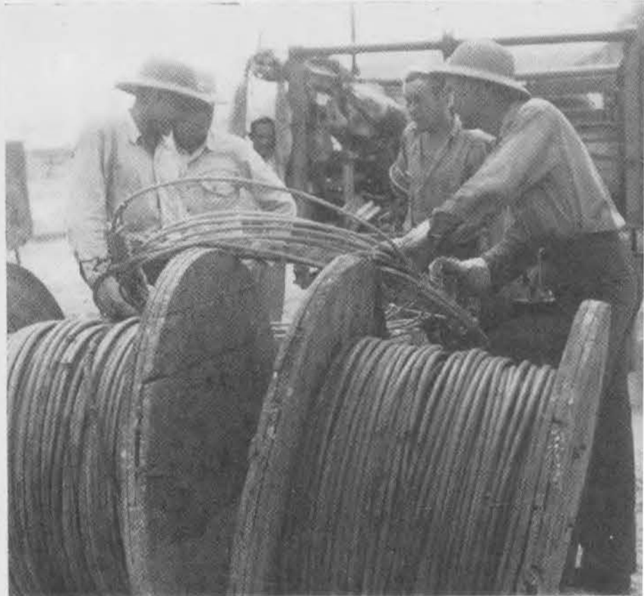
LINEMEN IN THE FIELD. Former Bell Telephone and hot-wire linemen now do the same type of work for the Navy. Miles of telephone wire and power cables were strung by these busy crews who seemed to revel in their work.
