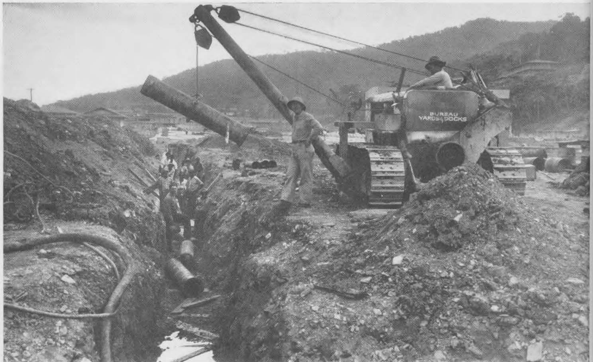
PIPE LINE GANG at work. Miles of pipe line were laid by this competent and active crew of Seabees and their native helpers. Modern war cannot be fought without oil and these men saw to it that our ships were amply provided with this necessity. Carpenter Abner F. Johnson of the 83rd, directs the lowering of a section of 20" pipe into the trench.
