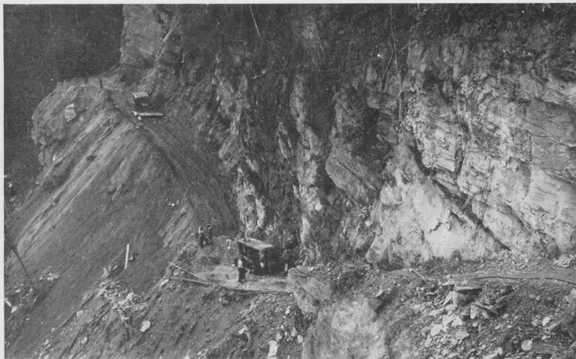
SCENE ON MARACAS ROAD. Just to look at the surveyors' line made experienced road builders paw the air and shriek in agony. 7.3 miles not only through the mountains but over them. At one time, the Seabees were using 5,500 pounds of dynamite per week. Fighting time and deadly avalanches which destroyed heavy equipment and cancelled weeks of hard labour; in spite of heights, gaps and the difficulty of moving heavy equipment, the Seabees finally chiselled, blasted, ground and forced their way through. Today the road is a paved scenic highway and the maximum grade anywhere along its length is ten per cent.
