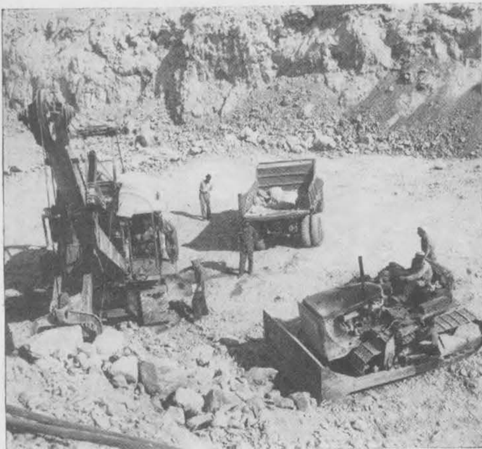
THE QUARRY. Daily, our drillers and blasters gouged at the obdurate walls of the cliff to obtain the quantities of rock demanded by our New Construction program. Here trucks are being loaded by a power shovel.
