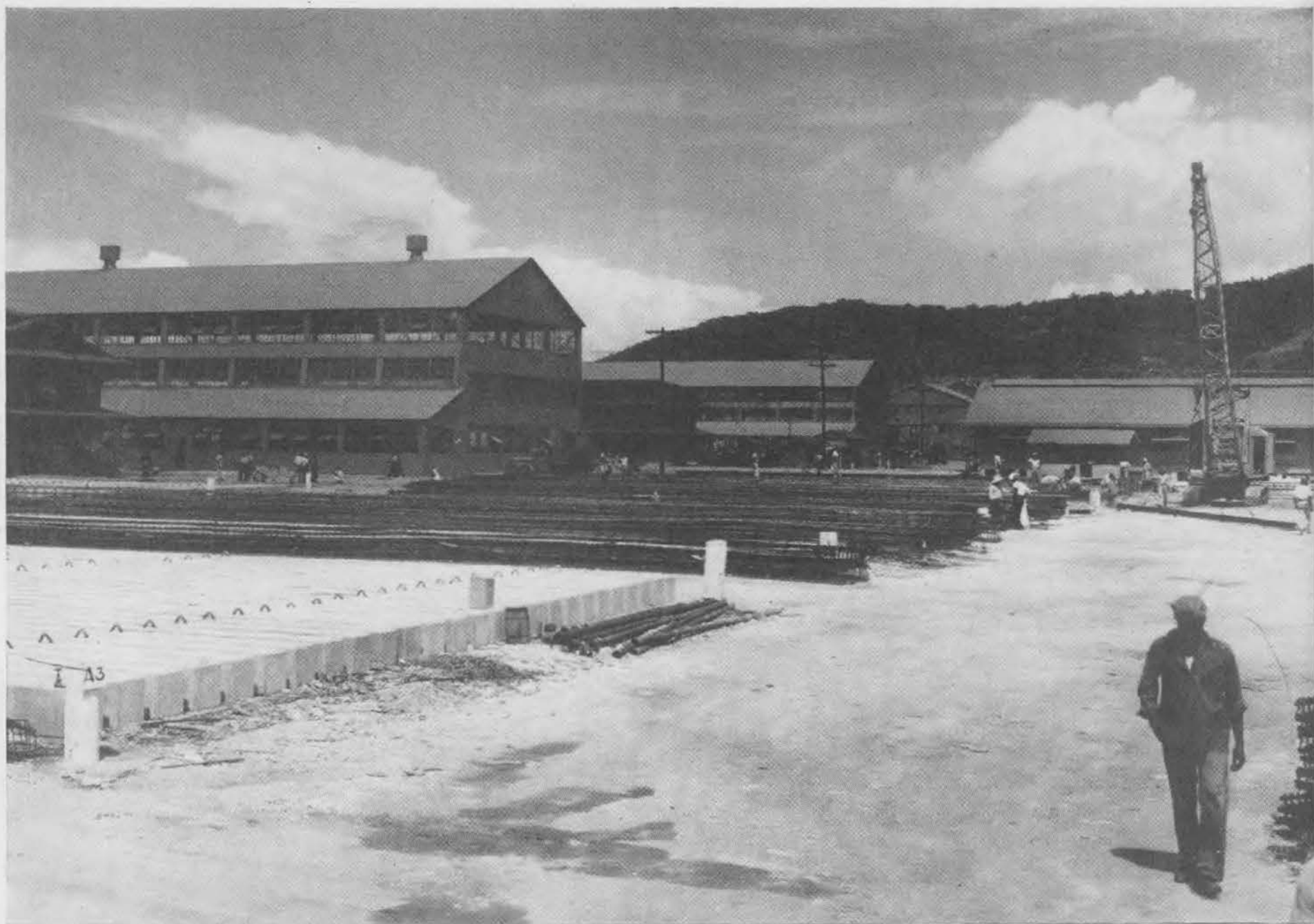
CONCRETE PILES used in the construction of N.O.B. piers are shown in left foreground. Each pile was 85 feet long and weighed approximately ten tons. Next to the piling is shown a rank of steel cages which were used to reinforce the concrete in the fabrication of the piles. Heavy duty crane in right background was used to lift and load these heavy units. In left background loom the N.O.B. Shops, which were completed and equipped by Seabees of the 83rd Battalion.
